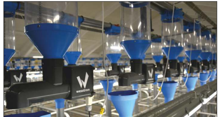
electric feed dispensers in the mating sector
